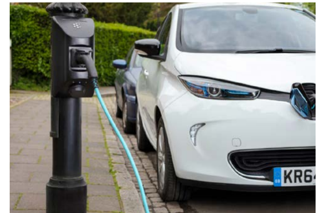
Figure 96: Example of on-street electric vehicle charging points.
