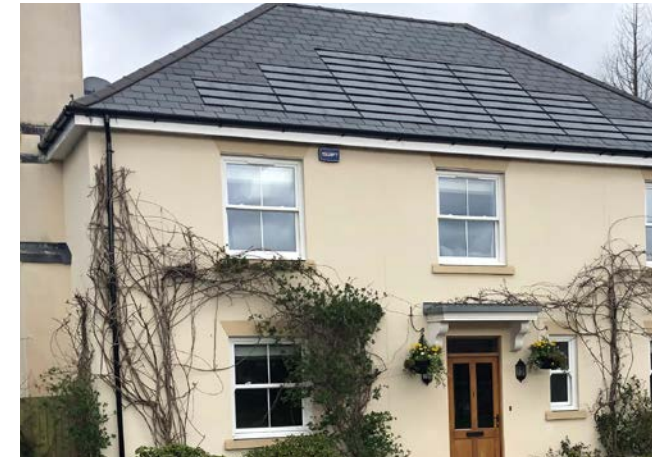
Figure 131: Use of single-like solar panels on a slate roof with the design and colour of the panels matching those of the adjacent slate tiles
